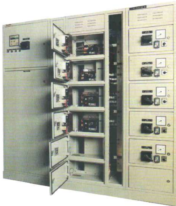
TYPICAL LV ELECTRICAL POWER DISTRIBUTION PANEL
